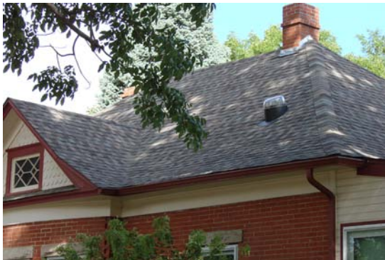
Appropriate solar "tube" installation
