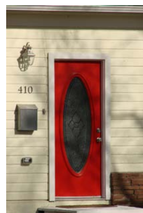
Inappropriate replacement door
