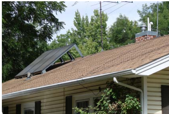
Inappropriate solar panel installation
