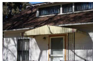
Inappropriate porch materials
