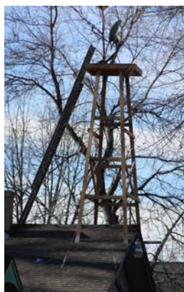
Inappropriate satellite dish installation
