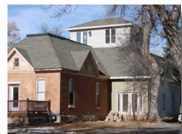
Inappropriate scale and massing of addition
