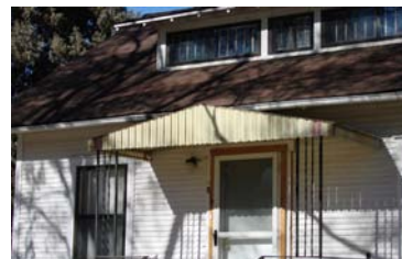
Inappropriate porch materials
