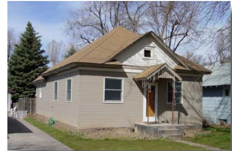
Inappropriate window replacement, where window openings have been reduced in size.
