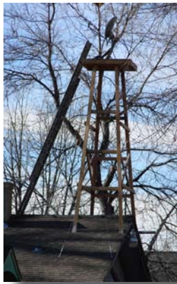
Inappropriate satellite dish installation
