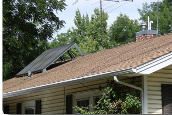
Inappropriate solar panel installation
