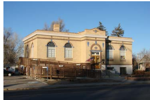
Inappropriate access that adversely impacts the historic character of the building's primary facade
