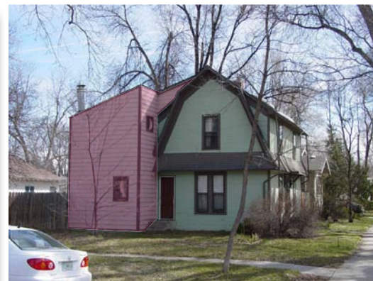
Inappropriate design, massing and roofline of addition
