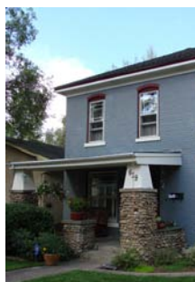
Inappropriate porch architectural style and materials
