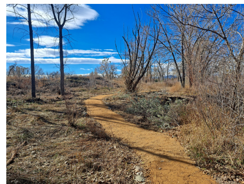
Boise Bend Trail erosion repair
