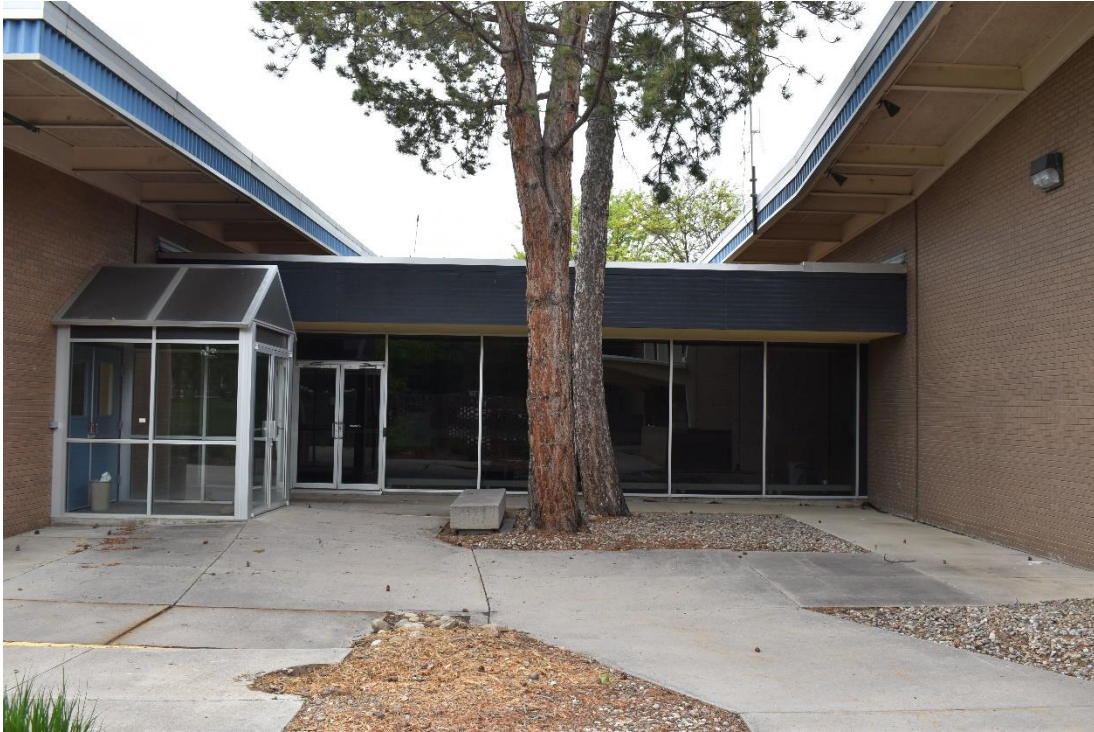
CD 1, Image 17, View to North, of the south side of the connector between Buildings B and C
