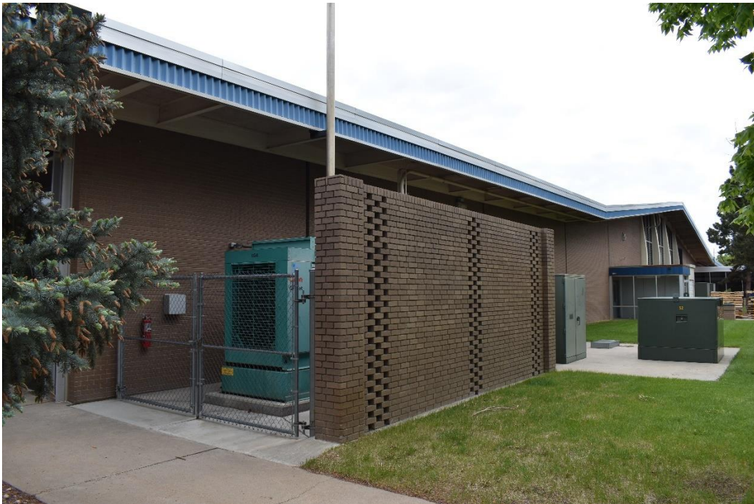
CD 1, Image 20, View to South-southeast, of the west wall of Building B
