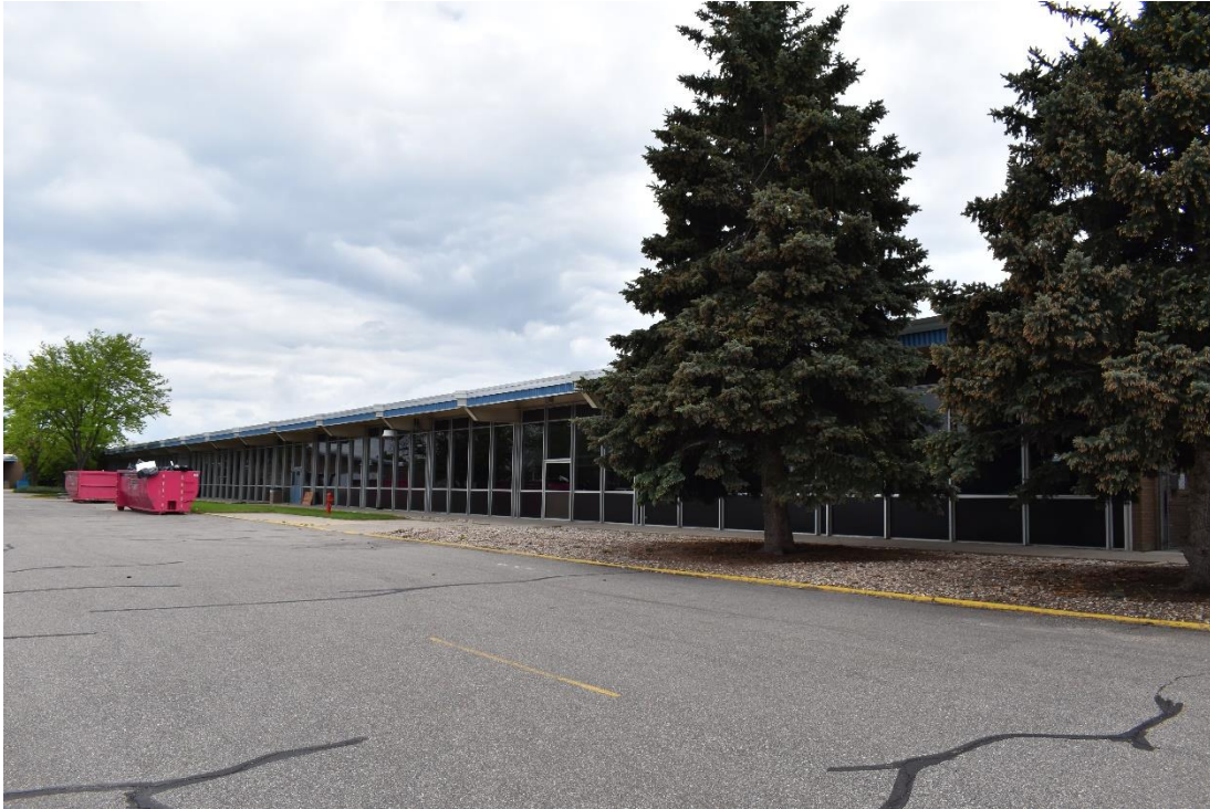
CD 1, Image 21, View to Southeast, of the north wall of Building B
