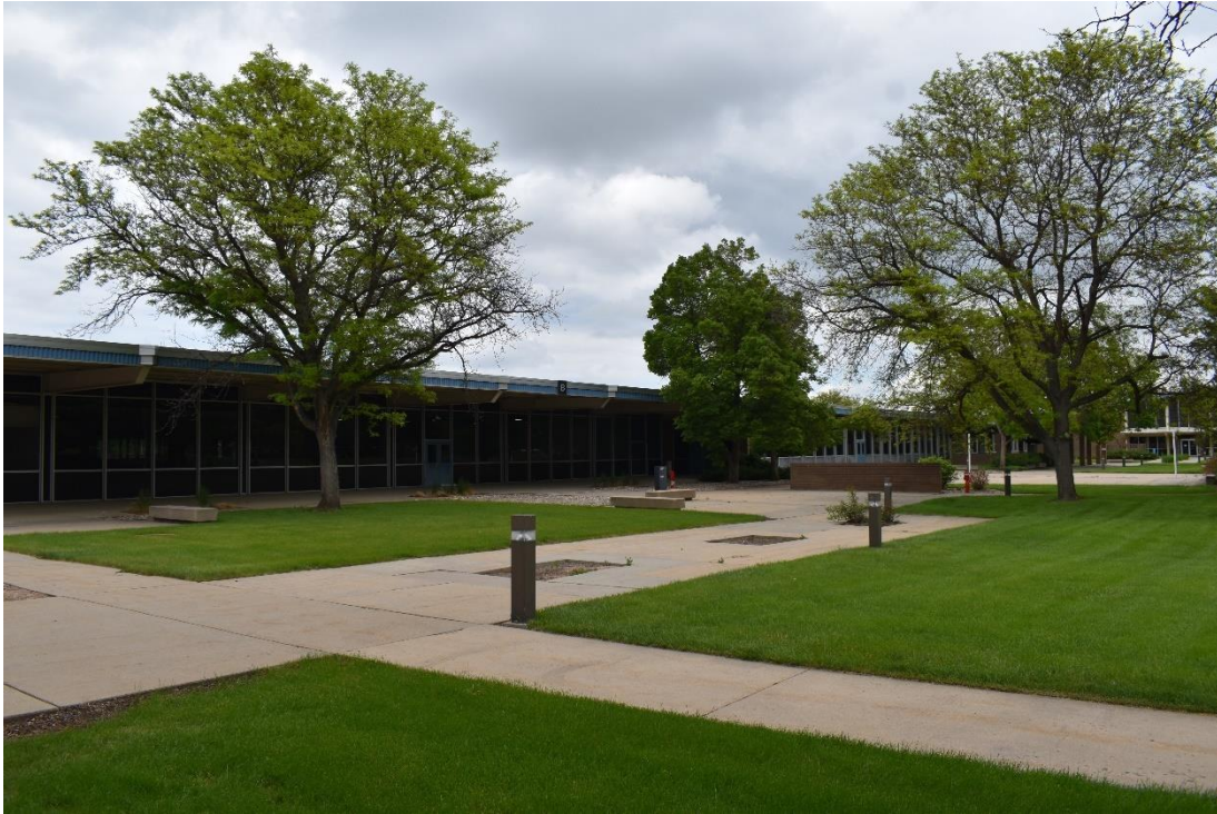
CD 1, Image 13, View to Northeast, of the south wall of Building B
