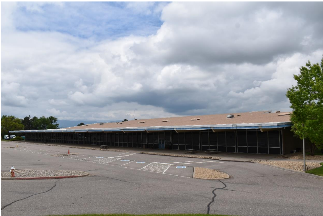
CD 1, Image 2, View to Northwest, of the south wall of Building A
