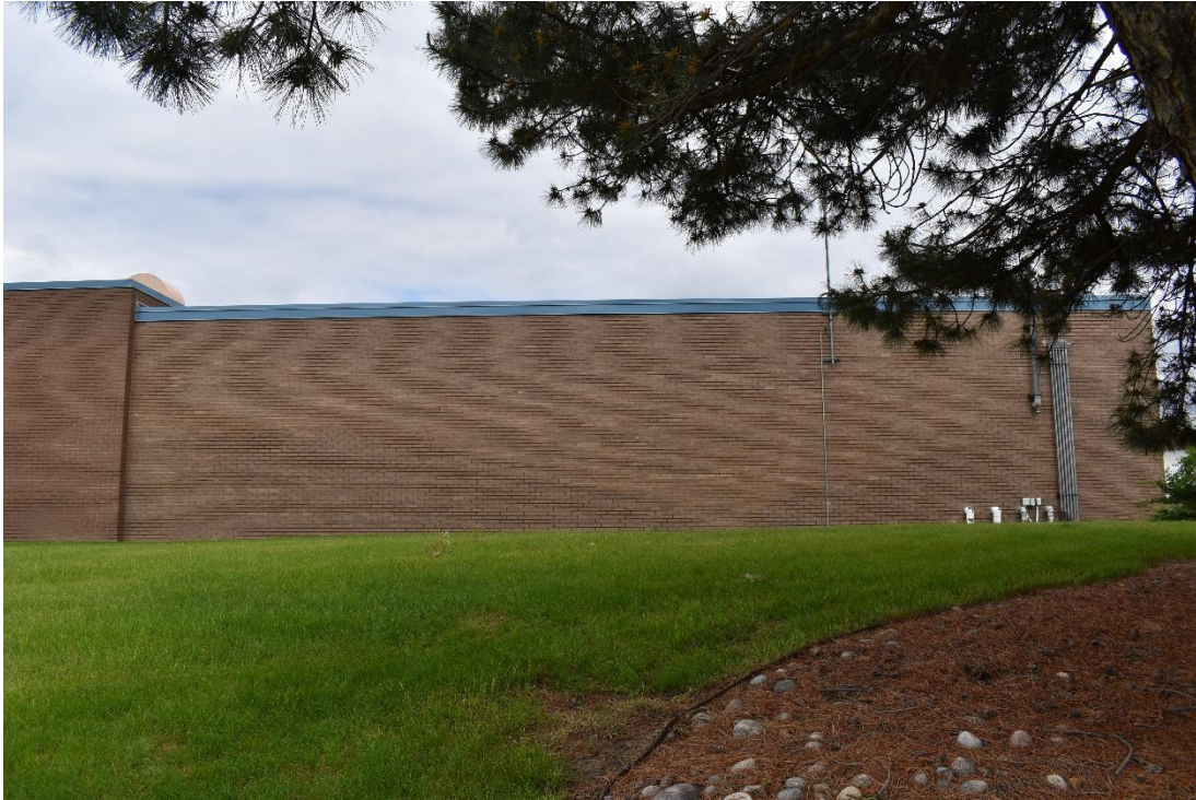
CD 1, Image 55, View to East, of the west wall of the Grounds Maintenance Building
