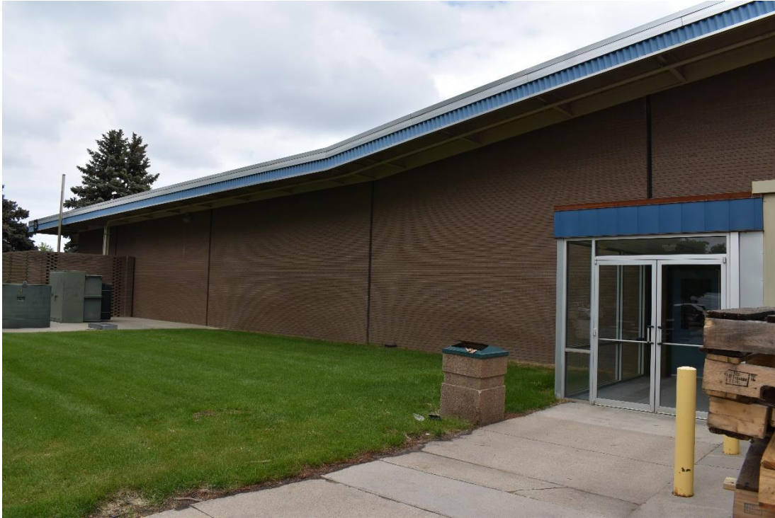
CD 1, Image 19, View to Northeast, of the west wall of Building B
