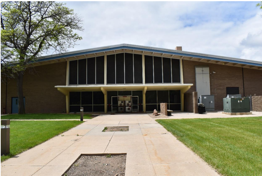
CD 1, Image 4, View to West, of the east wall of Building A
