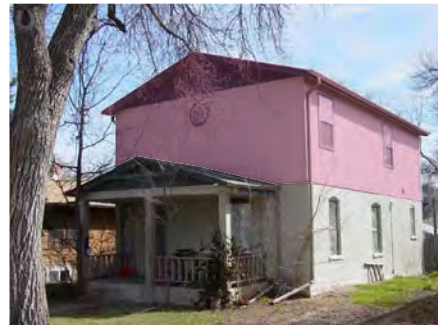
Inappropriate design and massing of upper level addition
