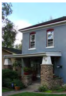
Inappropriate porch architectural style and materials
