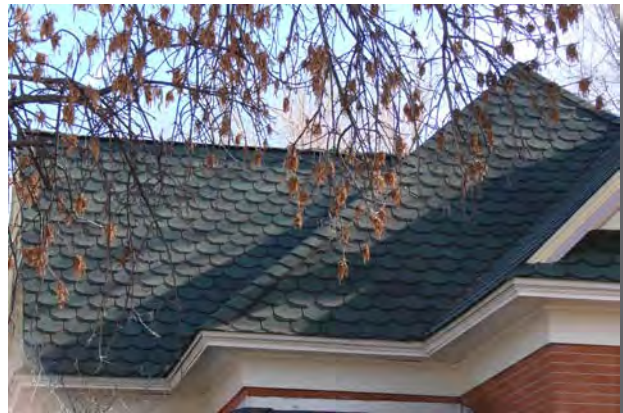
Inappropriate replacement fiberglass shingles in "faux" slate tile pattern
