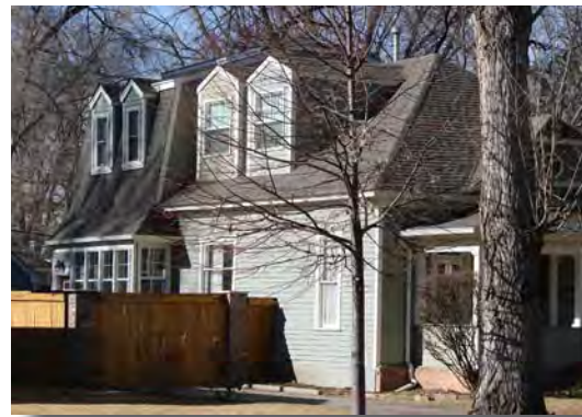
Inappropriate dormer design, massing and roofline
