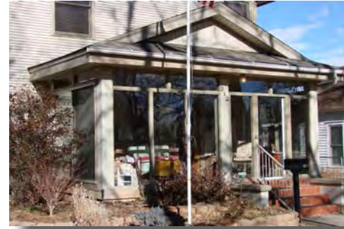
Inappropriate porch enclosure, with incompatible window style and sliding patio doors
