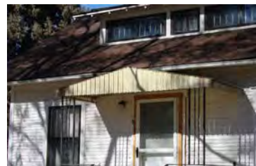
Inappropriate porch materials
