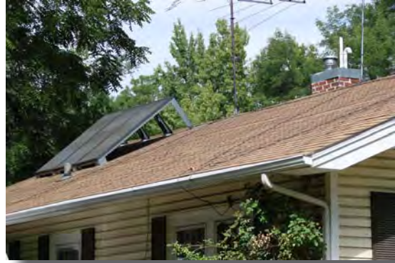
Inappropriate solar panel installation
