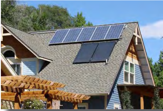
Appropriate solar panel installation, on rear roof shielded by dormer
