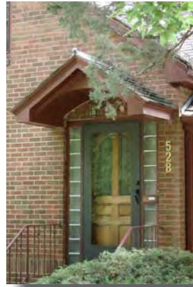
Appropriate storm door
