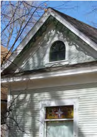
Narrow profile wood bevel lap siding with wood corner trims, wide head trim at fascia and decorative scalloped shingles in gable end
