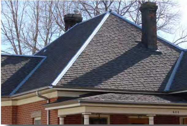
Appropriate replacement fiberglass shingles with metal hip and ridge caps, half-round gutters and round downspouts
