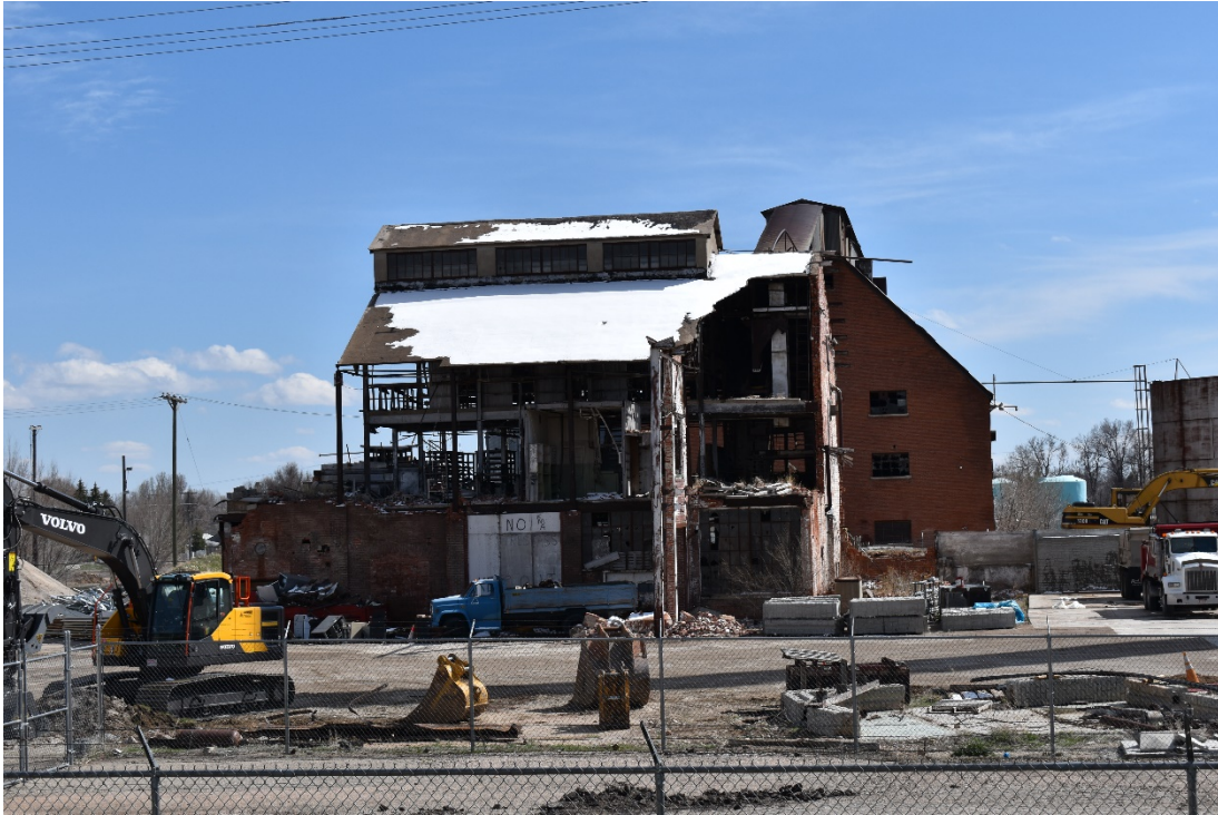
CD 2, Image 5, View to South of a section of a partially demolished building, and of a brick building. Photo taken from 11 th Street.
