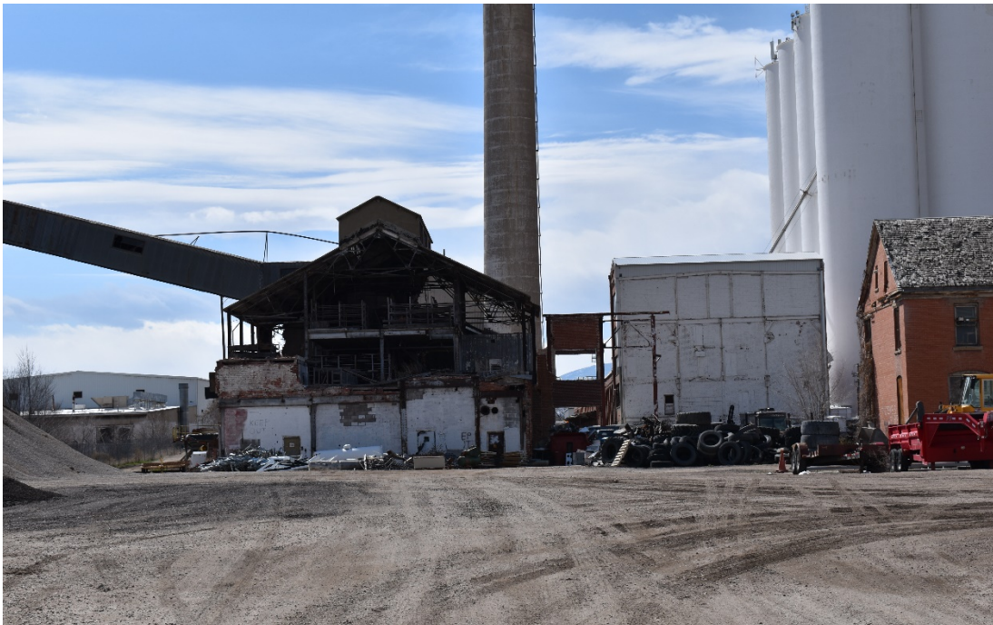
CD 2, Image 14, View to North, of a partially demolished building, the lower section of the smokestack, a steel structure, the concrete silos assemblage, and the southeast corner of the main office building. Photo taken from Madison Avenue.
