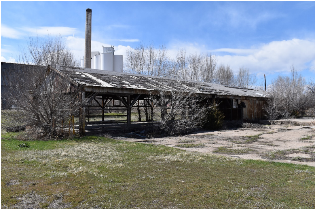
CD 2, Image 16, View to Northwest of a wood frame structure near the southeast corner of the property. Photo taken from Madison Avenue.
