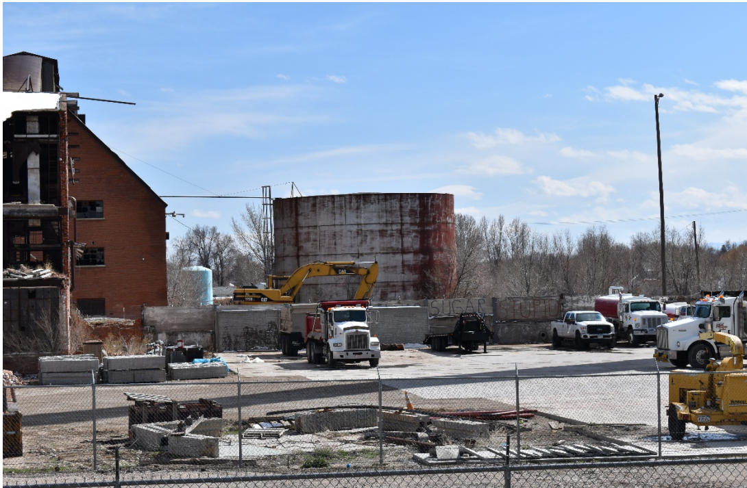
CD 2, Image 4, View to South of a round steel tank (used historically to store molasses syrup), a section of a brick building, and a section of a partially demolished building. Photo taken from 11 th Street.
