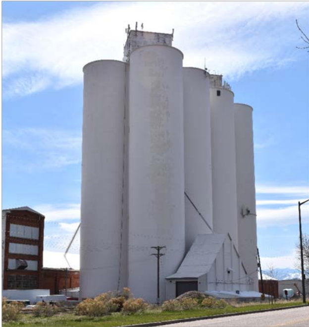
CD 2, Image 1, View to Southwest of assemblage of eight concrete silos, Photo taken from 11 th Street.
