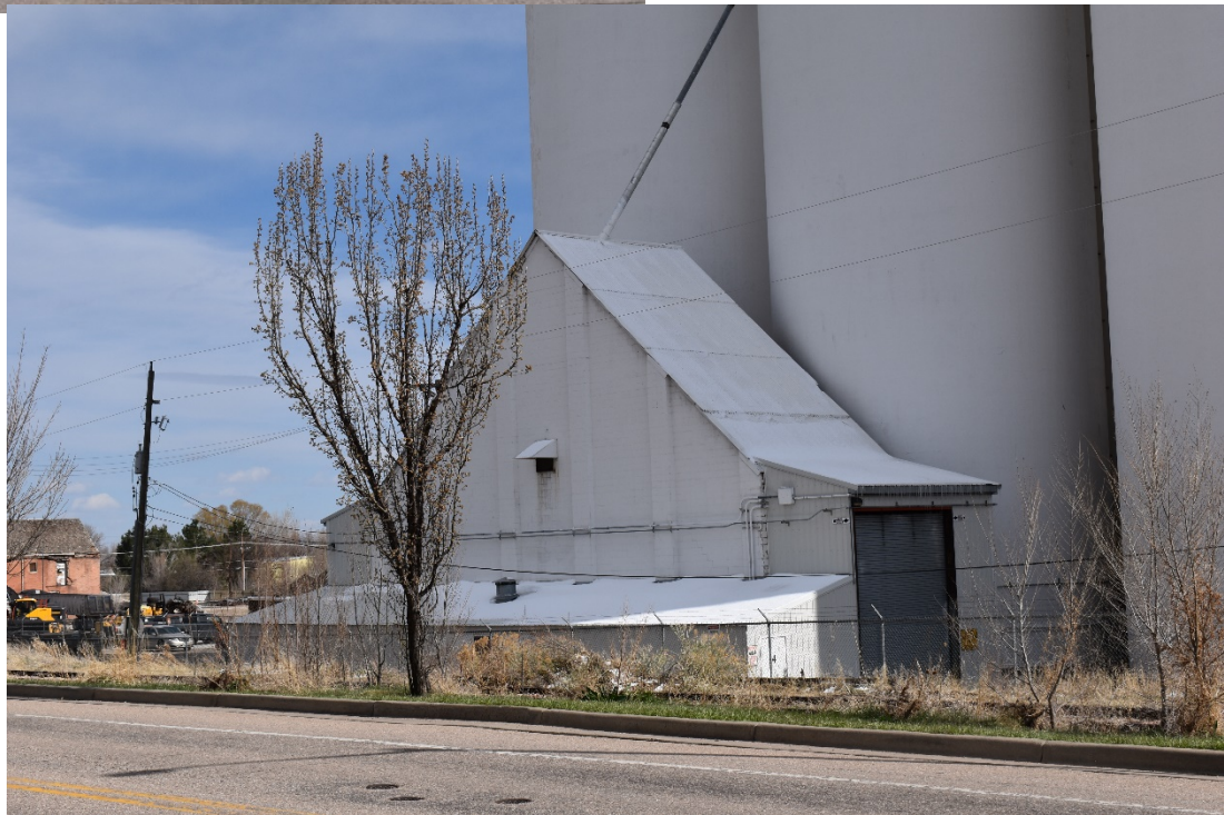
CD 2, Image 30, View to Southeast of the lower northeast end of the concrete silos assemblage. Photo taken from 11 th Avenue
