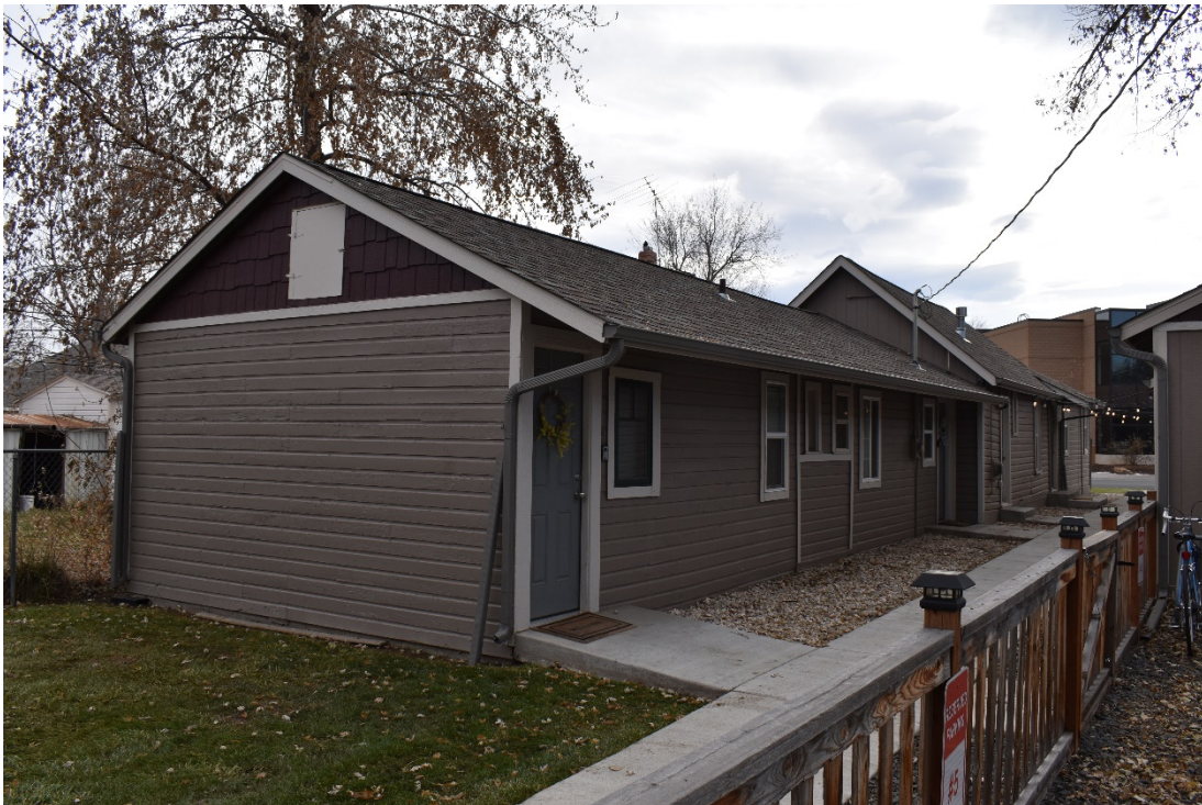
CD 1, Image 40, View to Southeast, of the north and west walls of the east building
