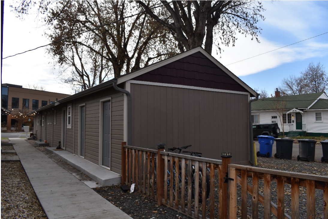
CD 1, Image 45, View to Southwest, of the east and north walls of the west building
