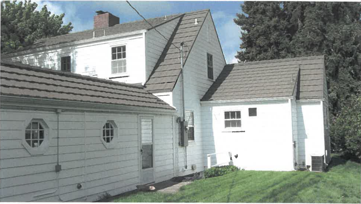
Photo 11: North side of house, 1953 side-gable addition and 1955 shed roof addition. Stairway to basement at corner where house and 1953 addition meet. June 2019.
