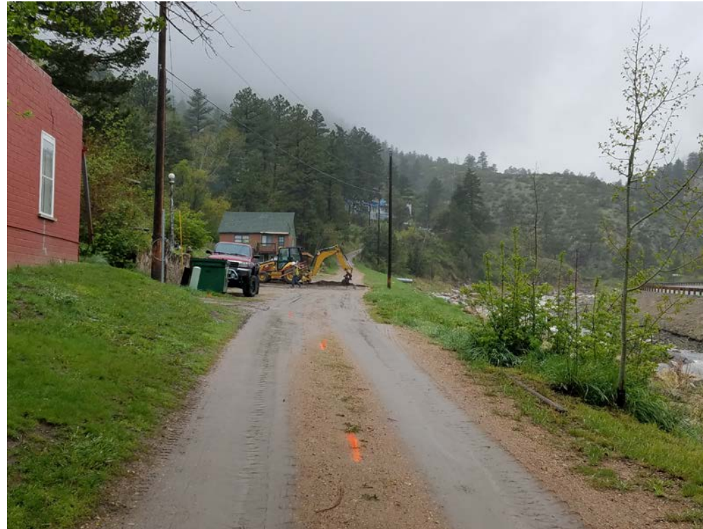
No pipe beyond dumpster
