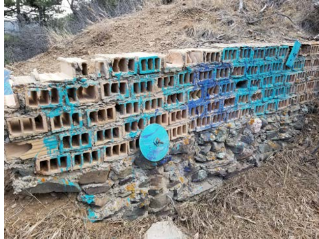
Vandalized Wall Near Surge pipe
