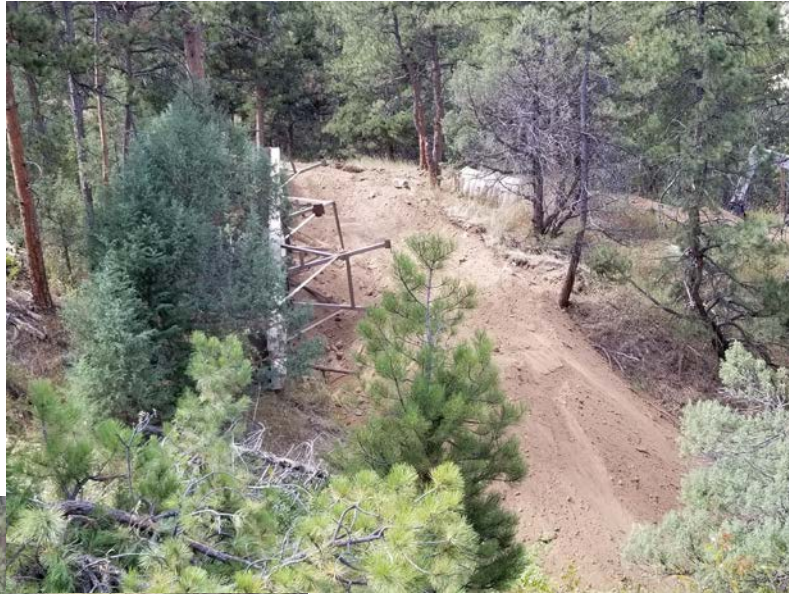
Pushed over Trestle and Pipe
