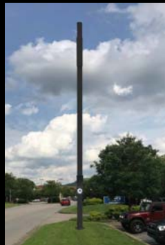
Small Cell Wireless Facility on stand-alone pole in ROW
