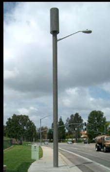
Small Cell Wireless Facility on utility street light pole in ROW
