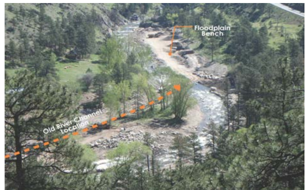
New river channel and floodplain bench to accommodate water when the river overtops
