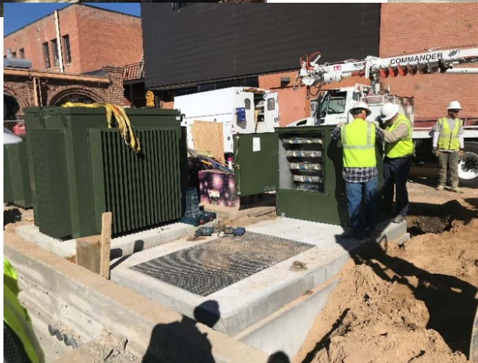
New transformer set that supplies power to the Rialto, Door 222 and the Mercantile
