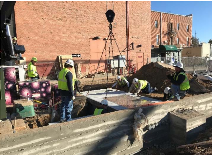
New electric vault set just north of the Foundry theater
