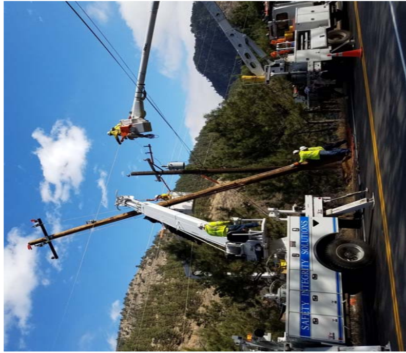
Inset of new pole between energized conductors along Hwy 34 near Cedar Cove
