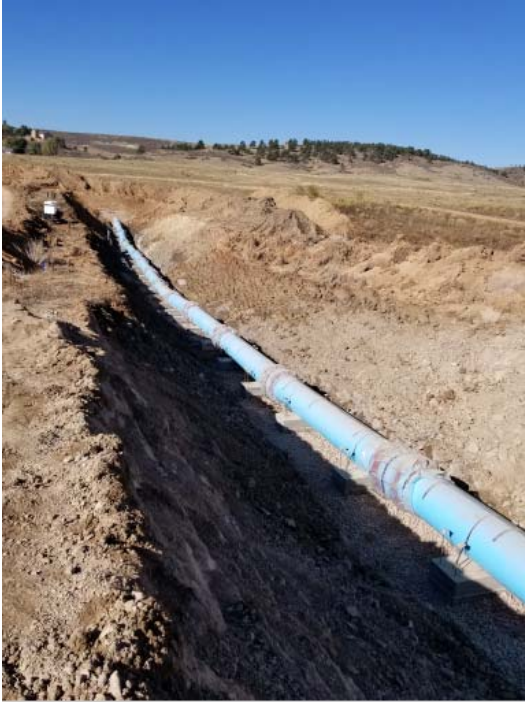
30" PVC water main
