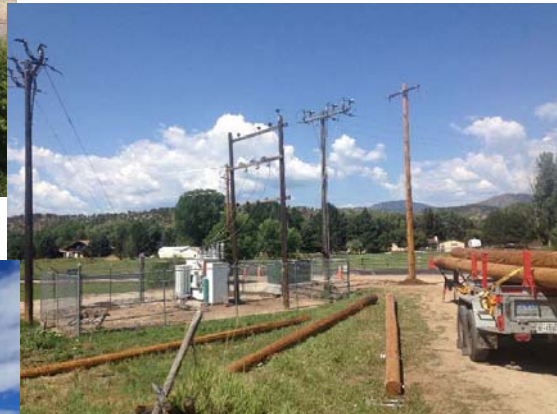
W3 at Cottonwood Substation along
