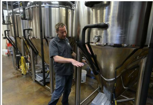
Josh Grenz, head brewer and co-owner of Verboten Brewing Co. in downtown Loveland, explains how the brewery's new 15-barrel fermenters work during a tour Tuesday of the company's new equipment. (Craig Young / Loveland Reporter-Herald)
