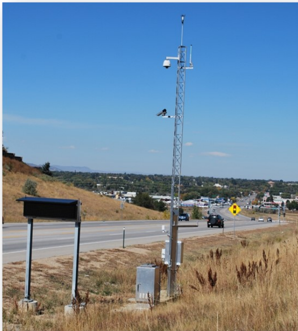
DERBY HILL WEATHER STATION/VMS – North-bound on US 287 South
