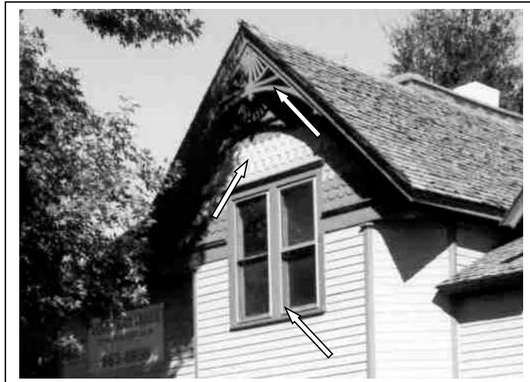
Photo #5. Gable ornamentation includes multi-colored patterned wood shingles, upper gable ornaments, and wood shingle roof. Also shown is a paired 1/1 double hung sash window.
