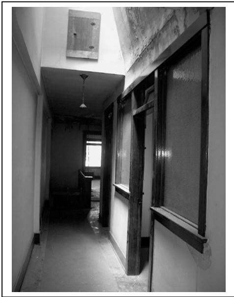
Photo #11. Upper level, interior hallway and one of several individual office-front entrances.
