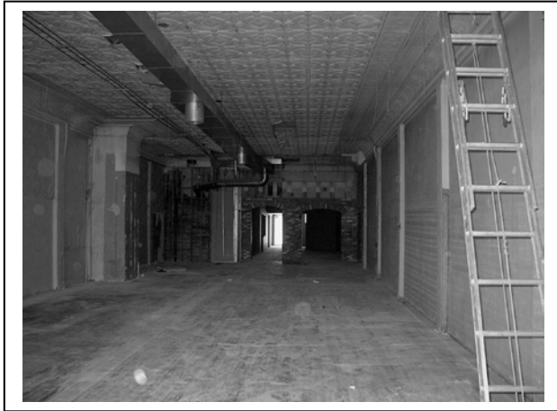
Photo #9. Building interior looking south. Two arched-passageways leading to the rear addition can be seen in the center of the picture.
