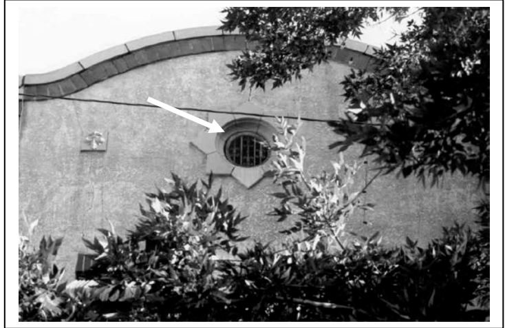
Photo #4. Oculus (circular) window with 8-point terra cotta star motif located on the gable of main façade.
