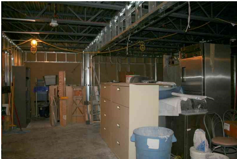
Interior view of the unfinished coffee shop area located on the main floor.
