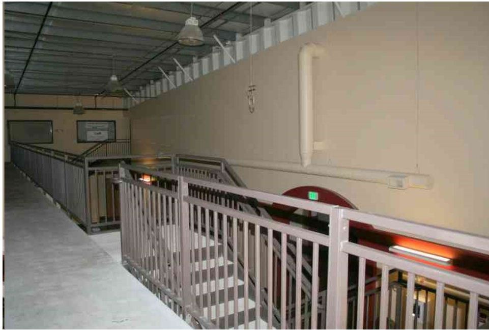
Interior view of a partially finished hallway/stairwell located on the second floor.
