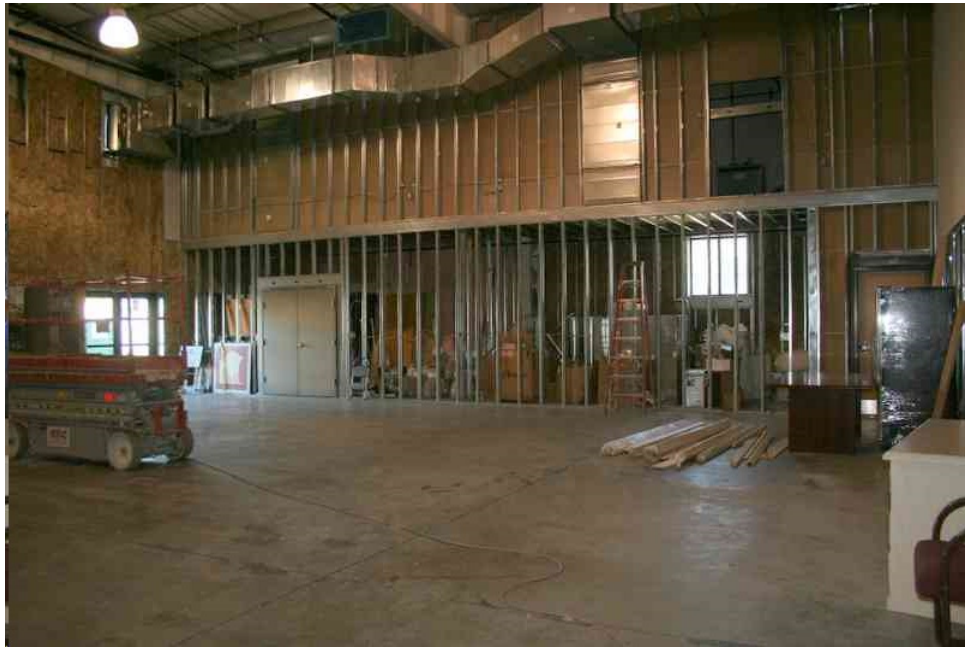
Interior view of the unfinished gym/performance area located on the main floor.
