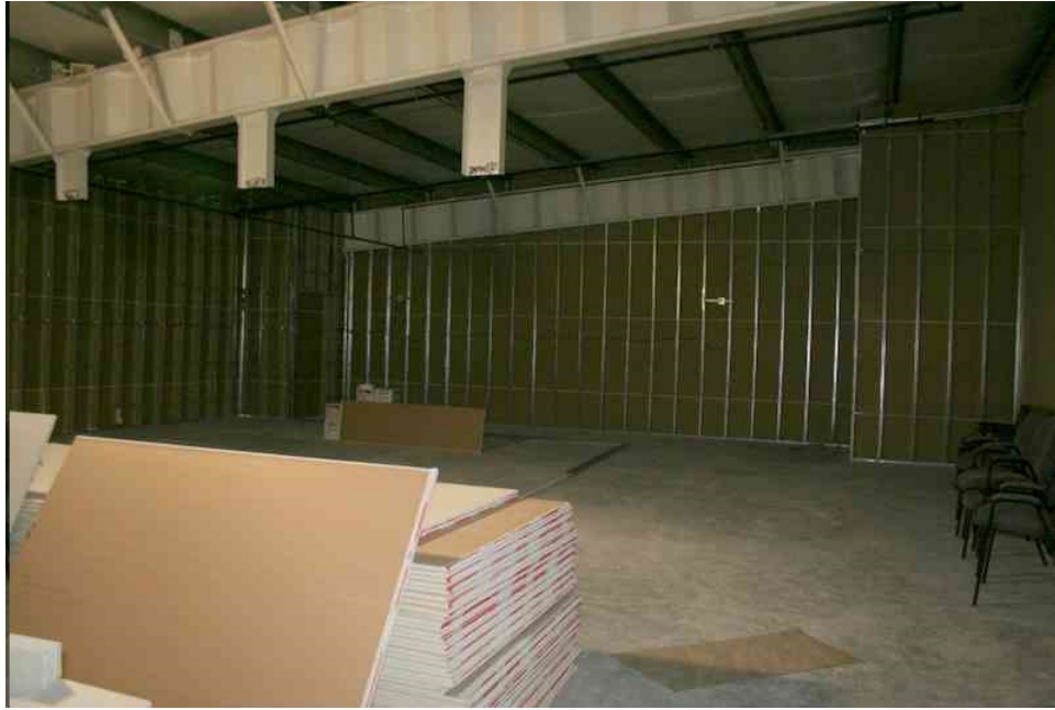
Interior view of an unfinished office area located on the second floor.
