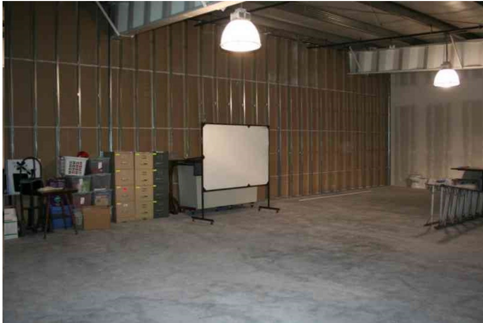
Interior view of an unfinished office area located on the second floor.
