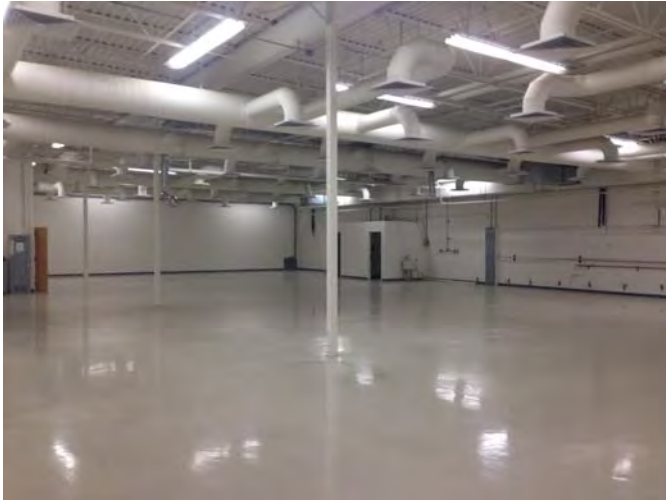
Switch room- main area.
