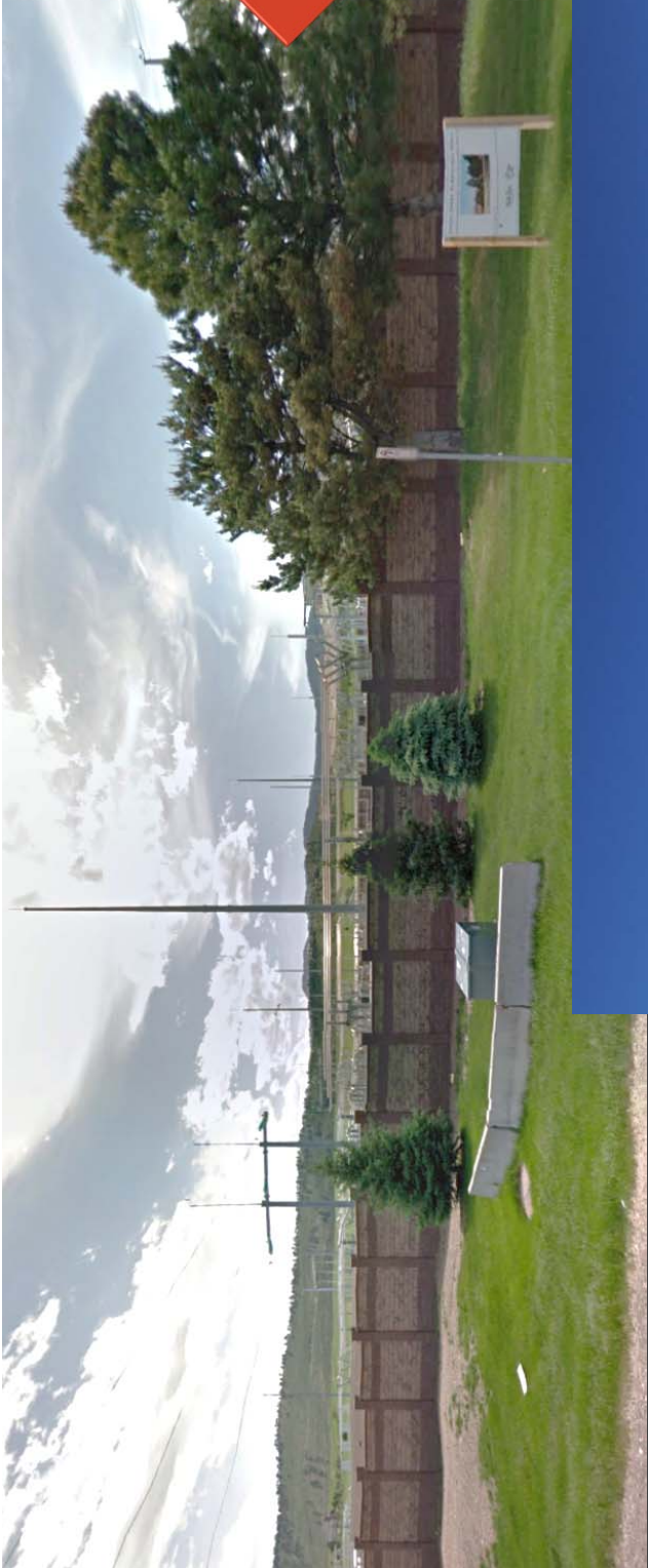
Dixon Creek Substation Fort Collins, CO Owned by Fort Collins Utilities and PRPA
