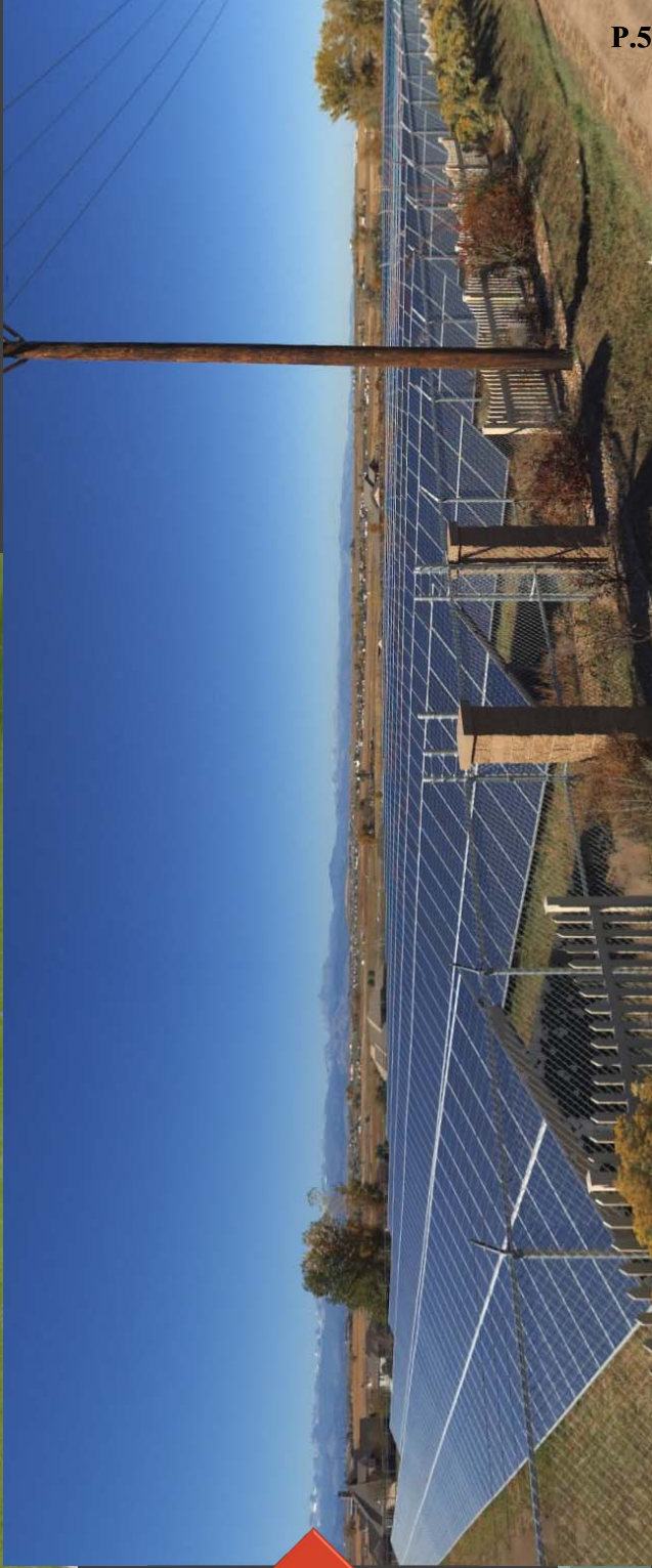
Hangar Solar Field Brighton, CO Owned by United Power 2MW Solar Field
