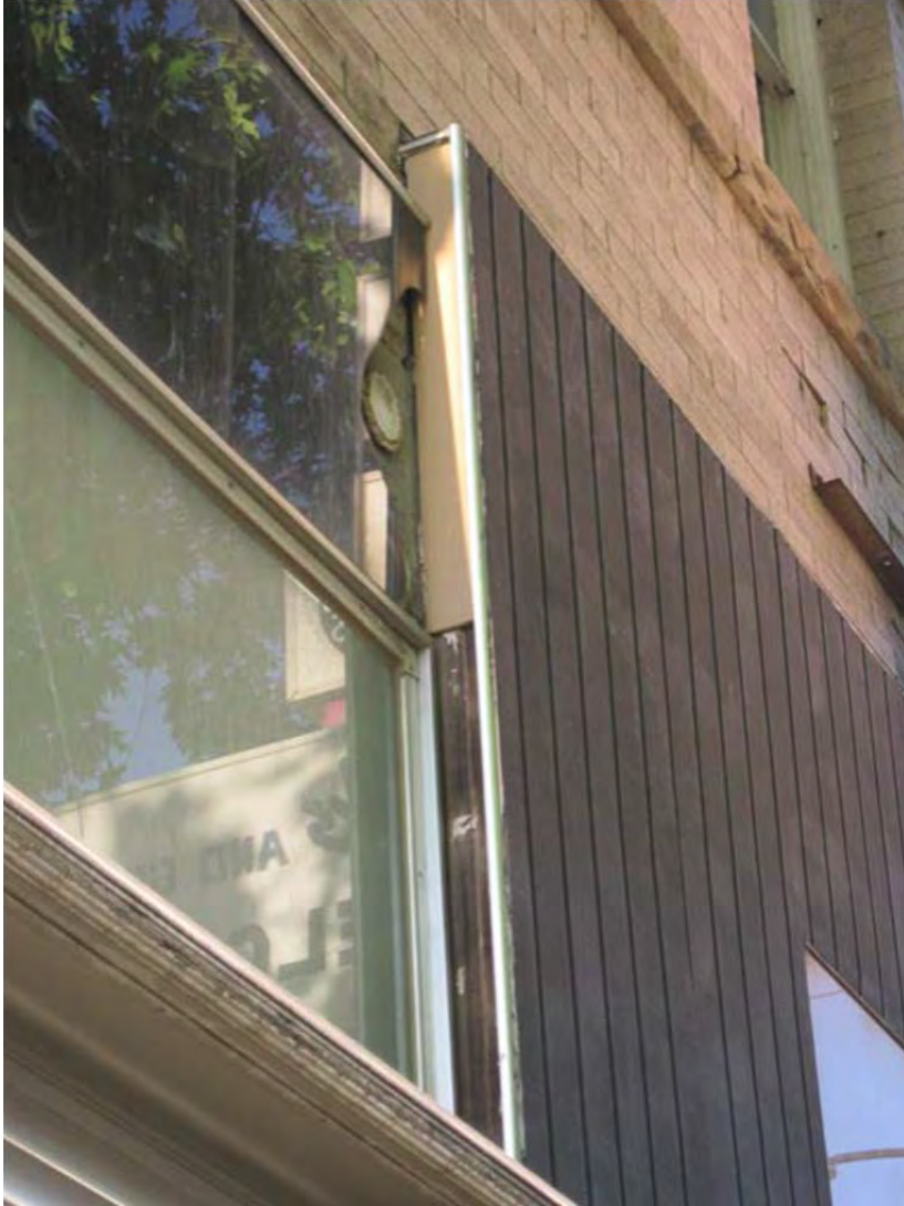
CLOSER VIEW OF CONDITION AT WEST EDGE OF SOUTH ENTRY FURRING
