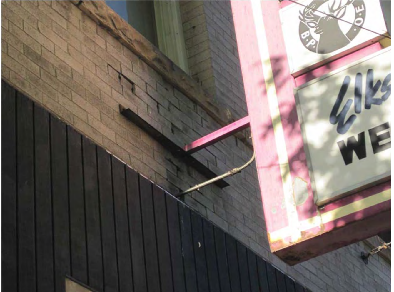
BRICK DAMAGE FROM PRIOR SIGN ATTACHMENT ON SOUTH ELEVATION ABOVE STOREFRONT
