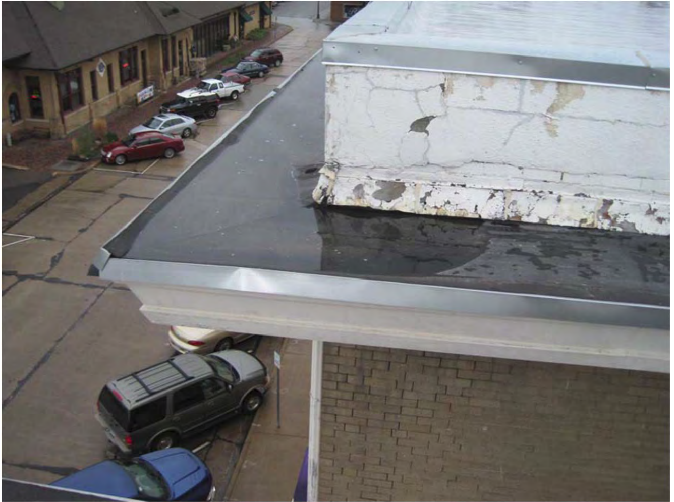
SOUTHWEST CORNER OF NORTH ROOF AT LIGHT WELL SHOWING SHEET METAL PARAPET CAP, PARAPET, MEMBRANE COVERED INTEGRAL GUTTER, SHEET METAL CORNICE, AND BRICK MASONRY
