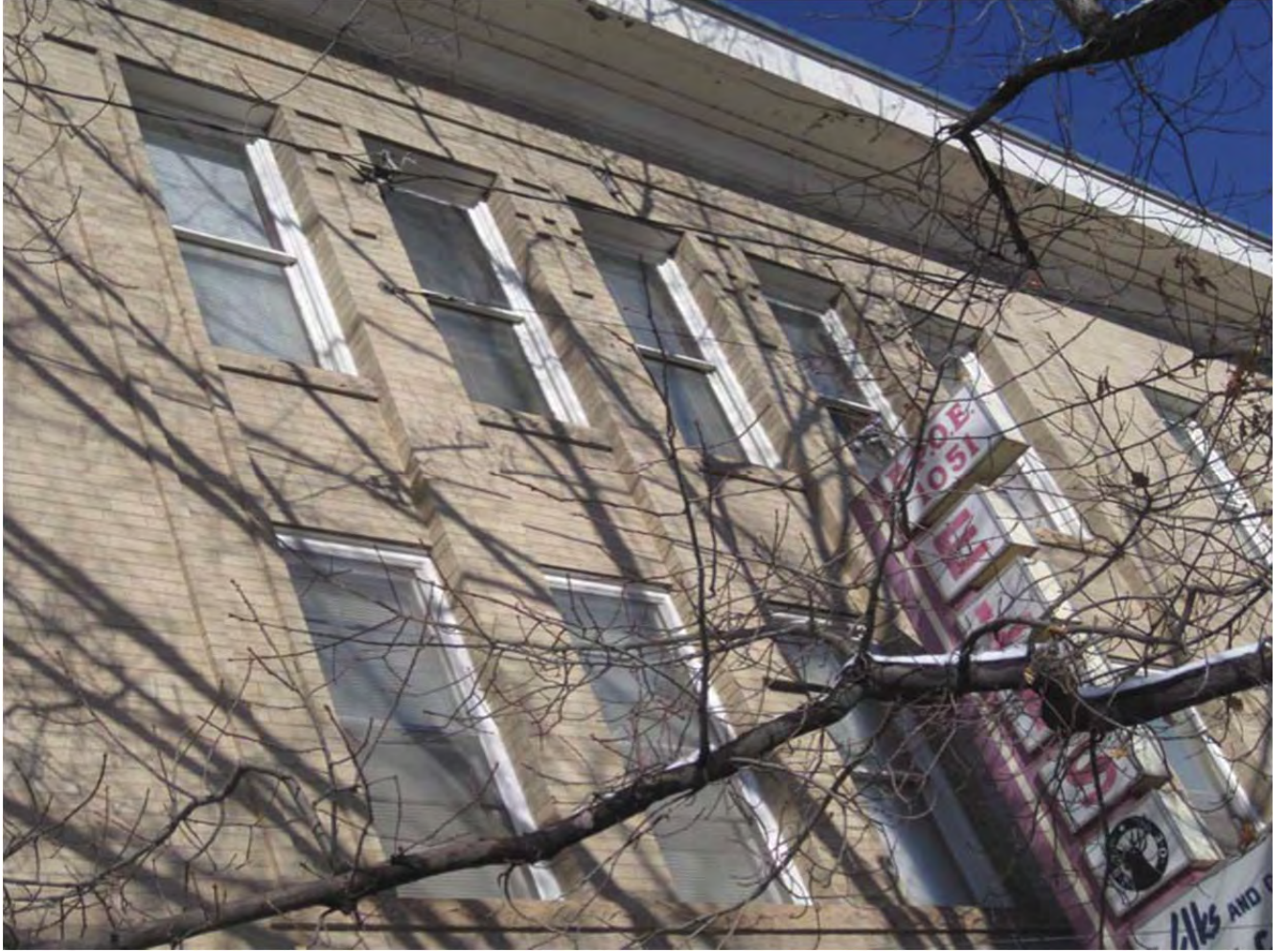
CENTER BANK OF SECOND AND THIRD FLOOR WINDOWS ON UPPER ORIGINAL SOUTH ELEVATION
