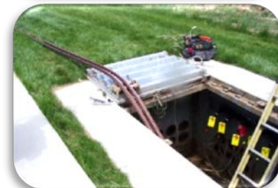
Power distributed through overhead & underground lines
