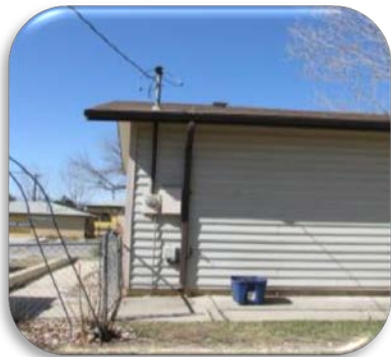
Power enters structures through service lines and usage is metered
