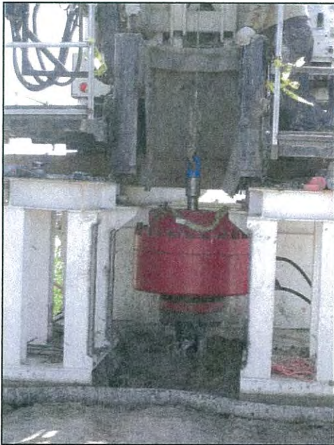
Figure C2. Photograph of blowout prevention (BOP) for annular space at base of drilling rig platform at MW02.
