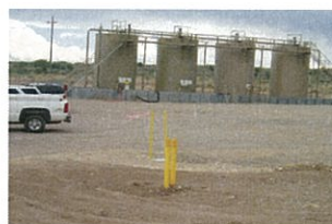
Each tank pictured is \approx 300bbl
