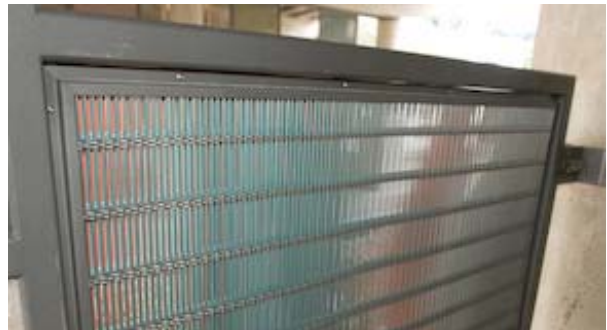
Figure 7: Unacceptable 50 percent open appearance
